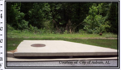
Stormwater curb inlet
